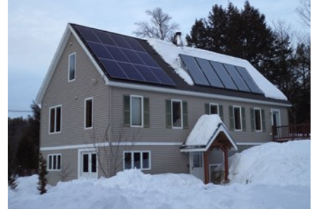
Photo: Roof mounted solar panels in New Hampshire, https://www.revisionenergy.com/solar-projects/wilmot-new-hampshire/
